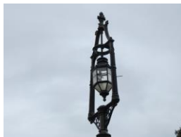
A Cause Celebre ! Heritage Lamposts- Victims Of Neglect Farncombe Road
